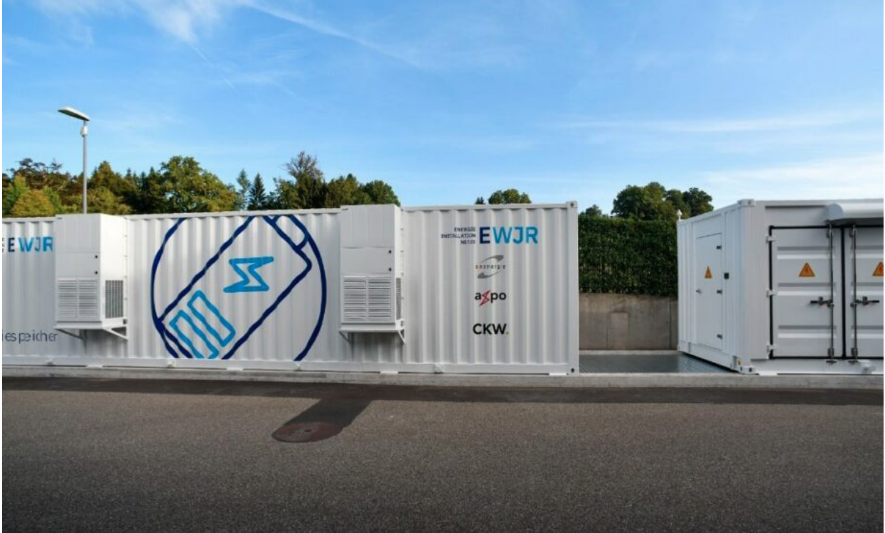
Axpo has already deployed a small battery storage project on home turf, this 2MW/2.17MWh unit at the Jona-Rapperswil power station
